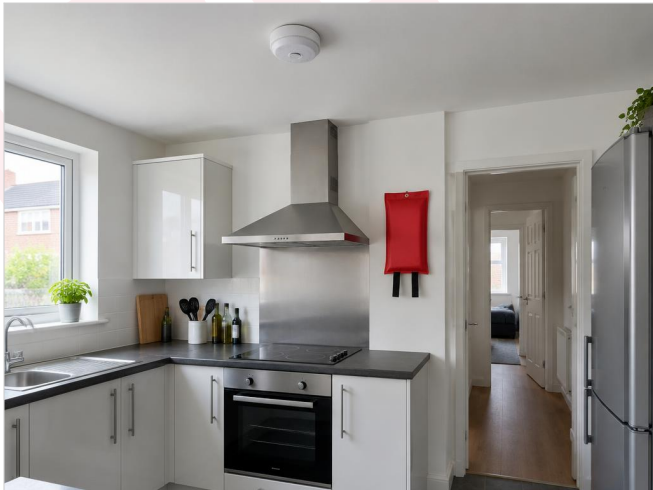
GREEN P04 · Kitchen heat detector and fire blanket (CX3, satisfactory)
