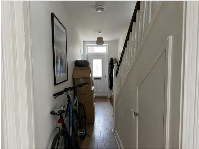
RED P02 · Bicycle and boxes in ground-floor escape route (ME1 → A1)
