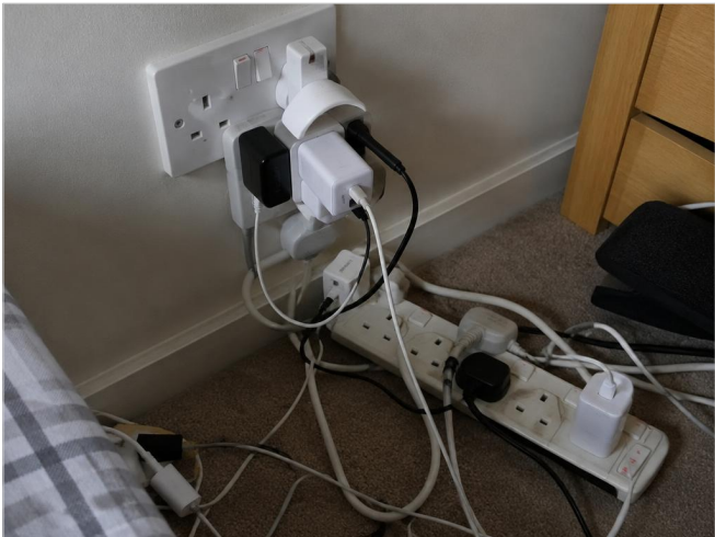
RED P03 · Daisy-chained extension leads, Room 3 (IG2 → A2)
