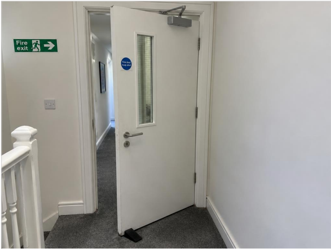
RED P01 · First-floor fire door wedged open (FDR1 → A1)
